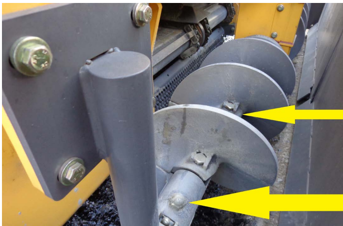
Set the augers so the head of material rises to the midpoint of the augers consistently across the width of the auger chamber. Photo courtesy John Ball of Top Quality Paving & Training
