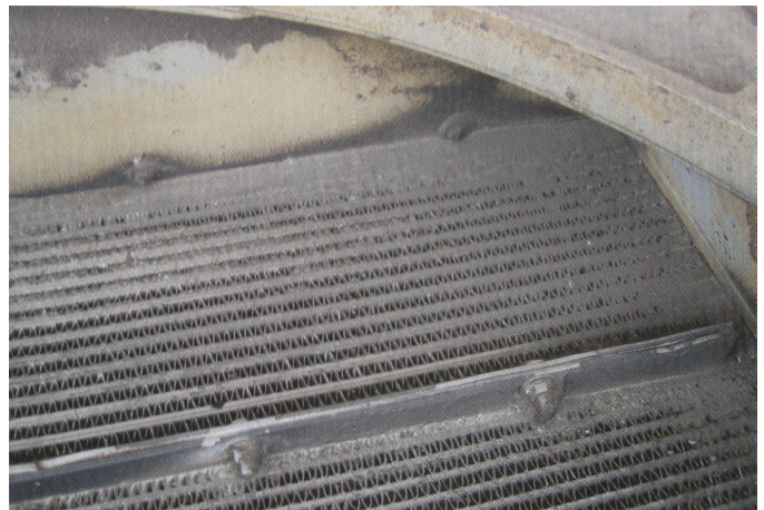
This dirty radiator can be cleaned by cooling the equipment down, using a citrus-based cleaner and then rinsing it with cool water.
